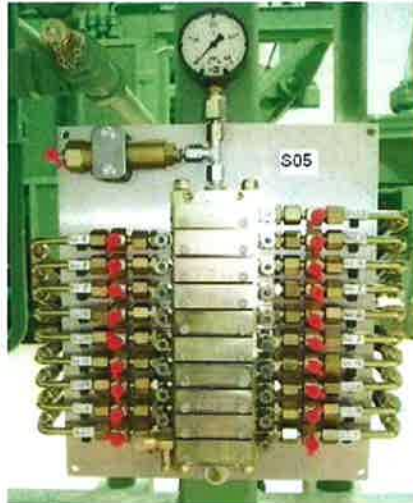
Distribution blocks located outside the safety fence for process equipment keep technicians out of hazardous areas while providing convenient access for one-point servicing.
